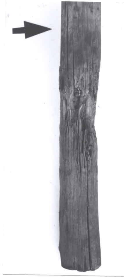
Fig. 1. A creosote-treated Eucalypt vineyard pole showing onset of premature failure below the (arrowed) ground line after 3 years of service under flood irrigation on the banks of the Orange River.
