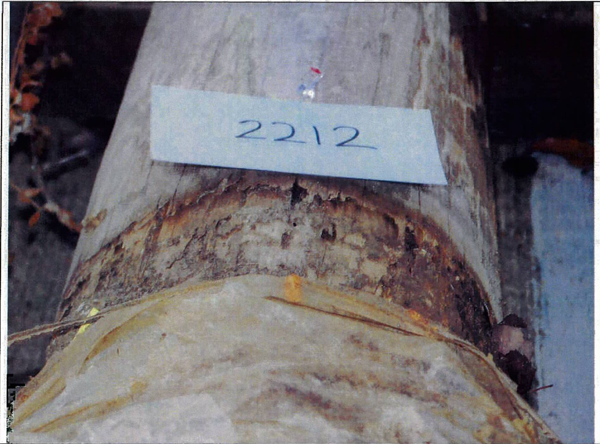
Figure 13 – Pole #2212 sustained the worst damage by termites in this study.
