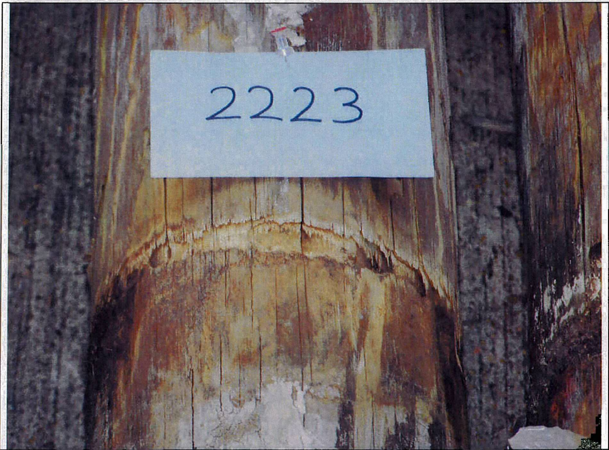
Figure 12 – Pole #2223 is an example of the type of termite damage found during this study.
