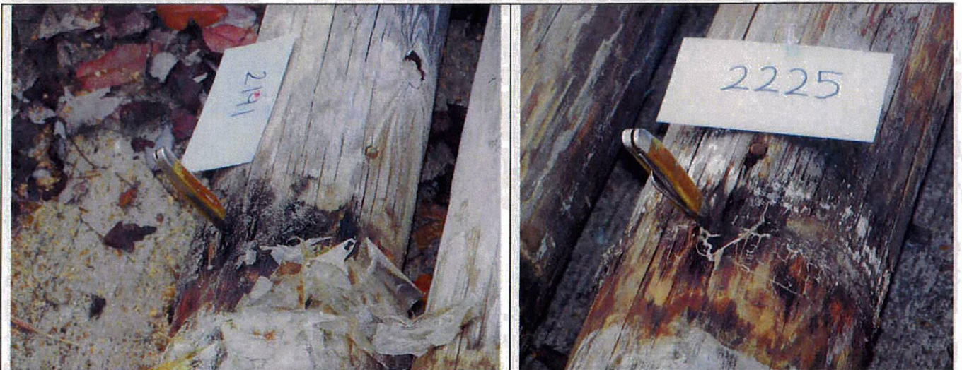
Figure 11 – A small pocket of deep decay was found on some poles.
