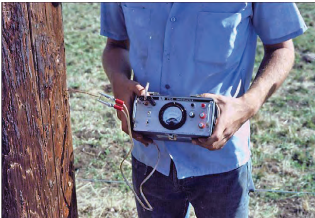
Figure 37. The Shigometer™ measures electrical resistance to detect rot in poles. Use an increment borer to determine the nature of the defect.
