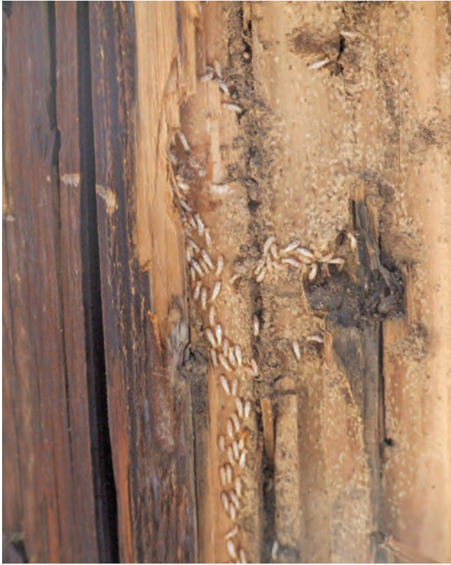
Figure 20. Example of termite damage to wood. Note the debris and termite excrement on the wood.
