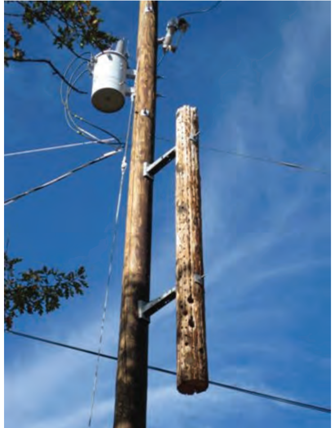
Figure 25. A section of old pole containing a woodpecker nest attached to a new pole in hopes of discouraging new attack.
