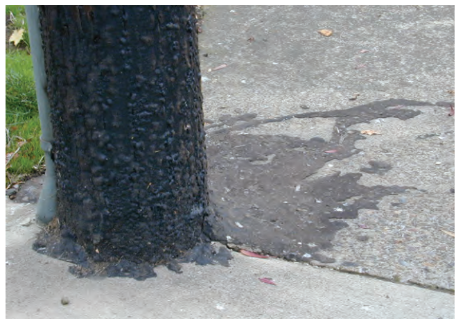
Figure 11. Example of bleeding from a creosote-treated pole.
