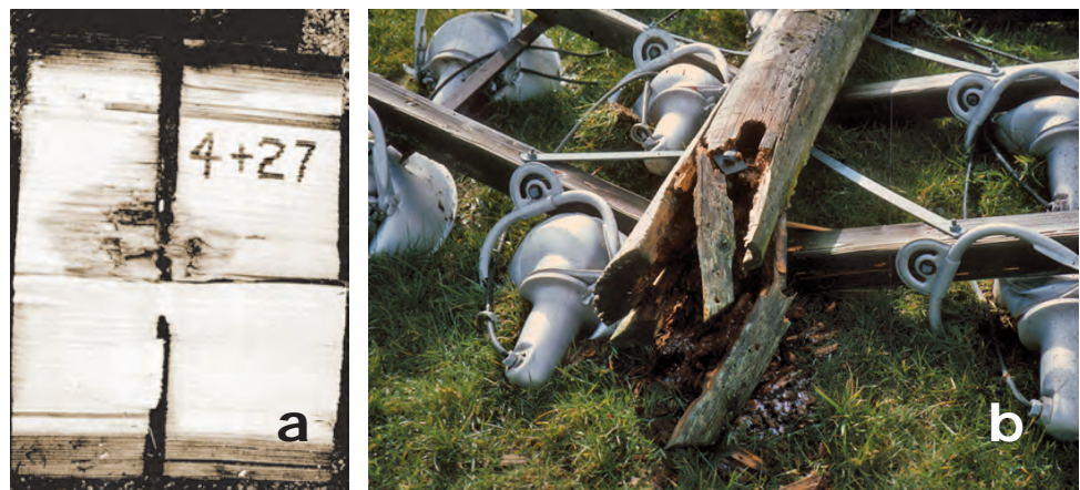
Figure 4. (a) Decay at the bolt hole and (b) pole failure caused by decay in a field-drilled hole.
